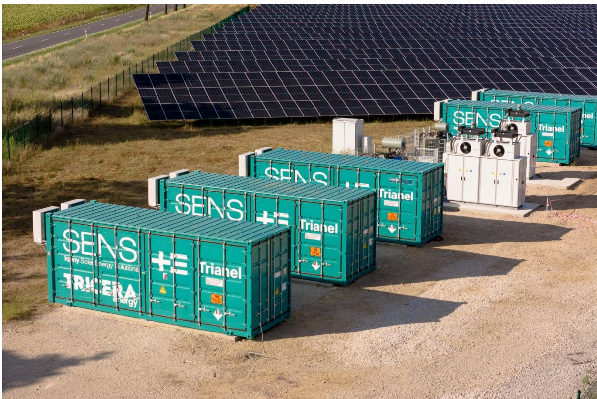
Photo: TRICERA energy's large-scale battery storage system from a project with Trianel in Lübars
