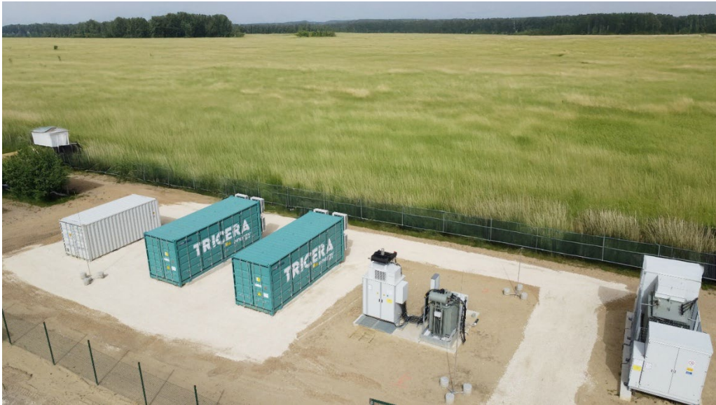
Picture: Symbolic image of a TRICERA battery storage system, as it is being built for SVS
