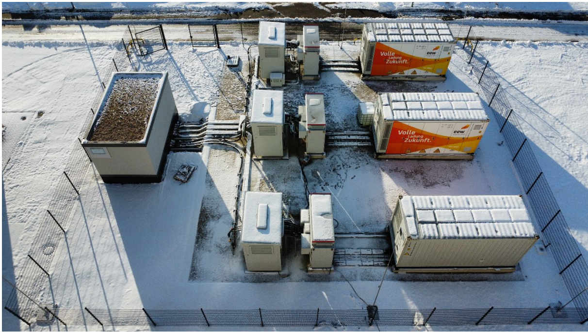
Image: Drone image of the TRICERA energy battery storage system on the EEW site in Premnitz
