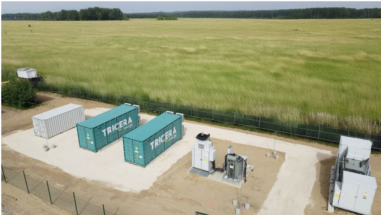
Symbolic image of TRICERA battery storage system, as it is being built for Ulm/Neu-Ulm municipal utilities
